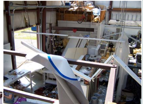
A garage door was blown in by the strong winds. Fallen debris litters the lab.
