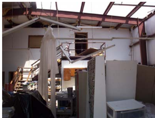
Twisted overhead lights hang below the missing roof section at Superior's Lab in Ocean Springs.
